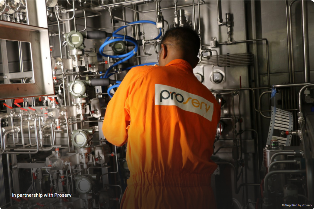
Proserv is a leading specialist in topside control solutions in the Middle East.
